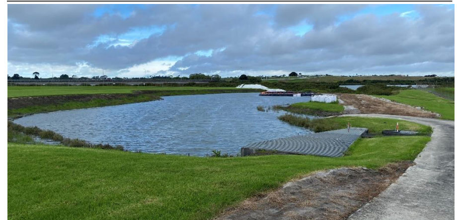
Upgrades to the stormwater system including an eastern airside stormwater pond, eastern arrivals forecourt, terminal enabling and Mānawa Bay precinct
